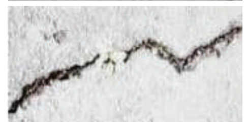
Fig.9: Concrete building cracking due to poor construction practice; water added to fresh concrete.
