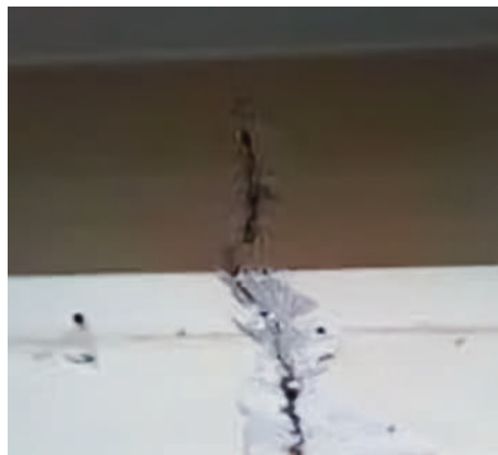
Fig.10: Major structural crack in beam due to poor detailing practice.
