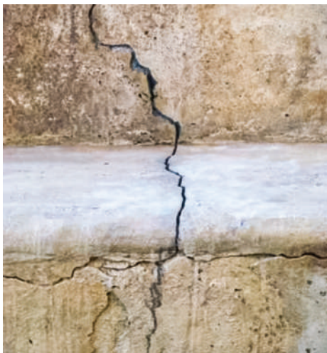
Fig. 4: Concrete building cracks due to creep movement
