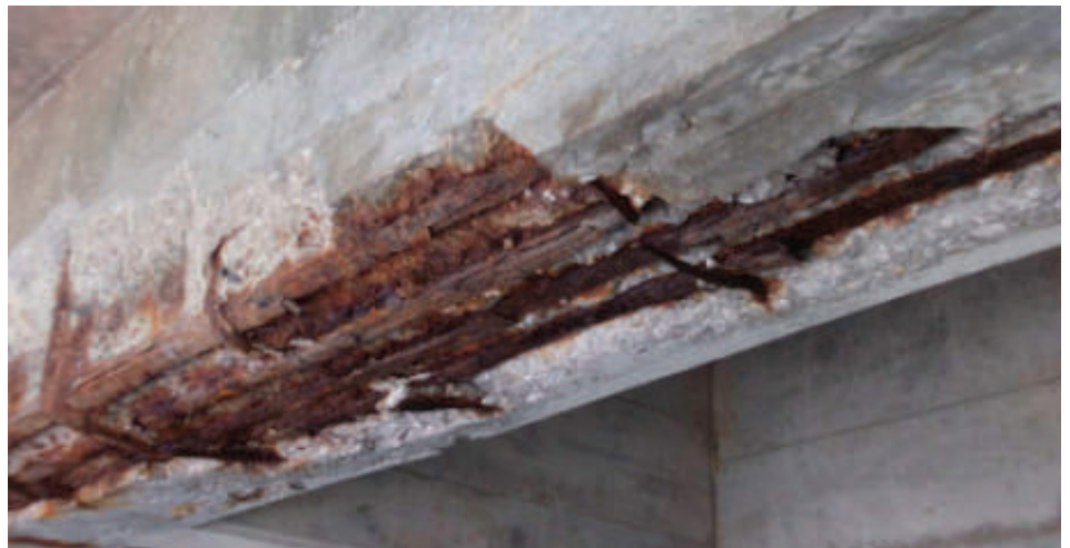
Fig. 5: Cracking due to corrosion of reinforcement
